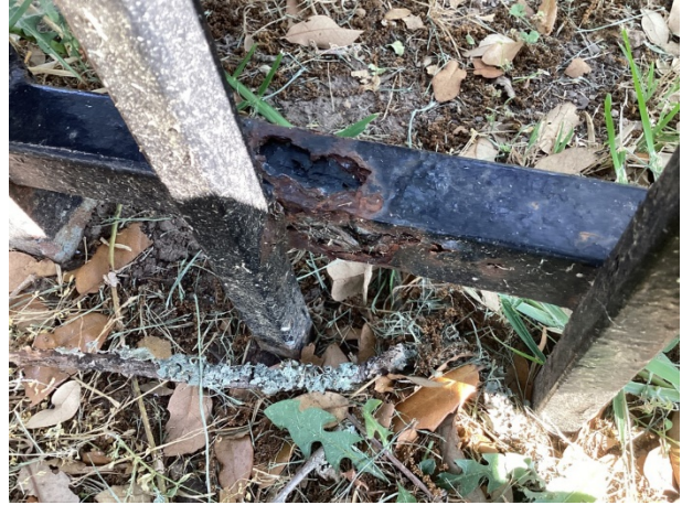
Fence damage and rust
