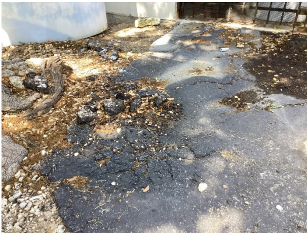
Pavement deterioration possibly caused due to tree roots
