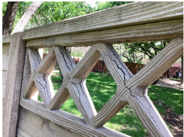
Cracks at lattice section
