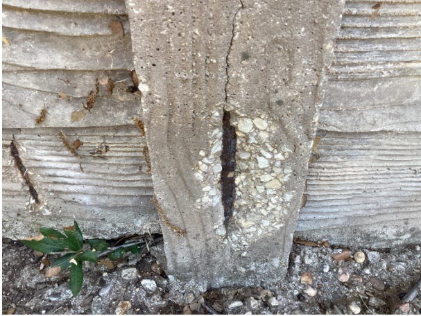
Concrete spalls and exposed reinforcing steel at column
