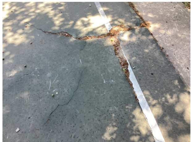
Surface cracks at basketball court
