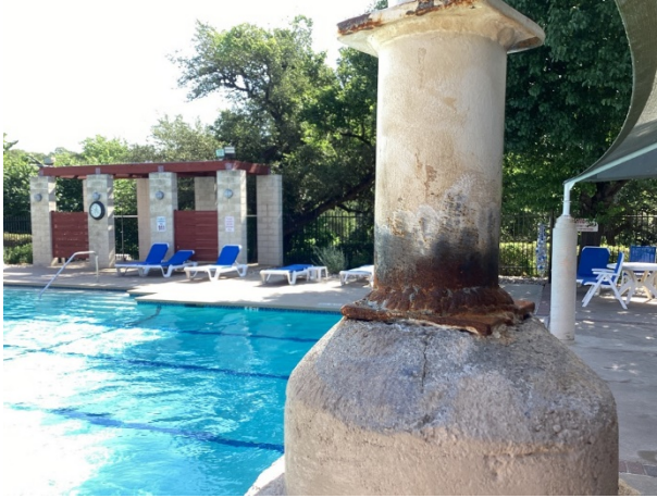
Rust at frame
