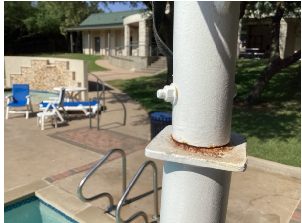
Rust at frame
