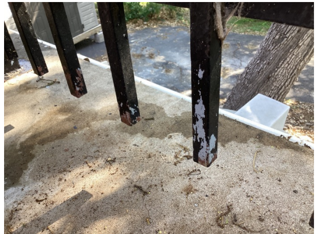
Fence finish deterioration and rust
