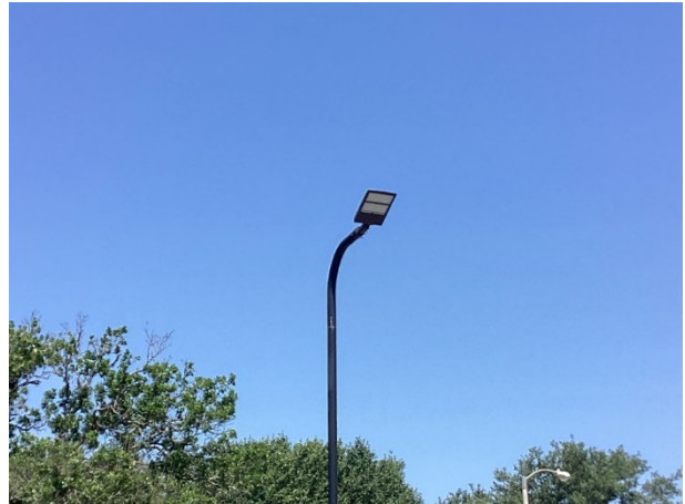
Recently replaced light fixture
