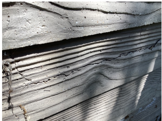
Wall panel cracks
