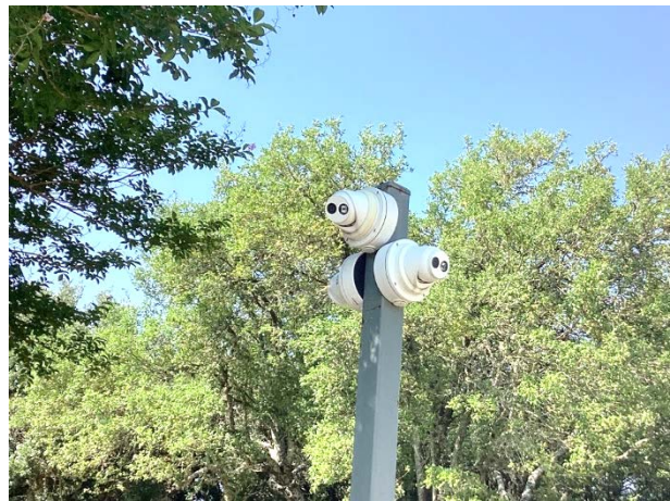
Security system cameras
