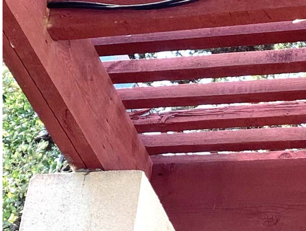
Pergola wood deterioration
