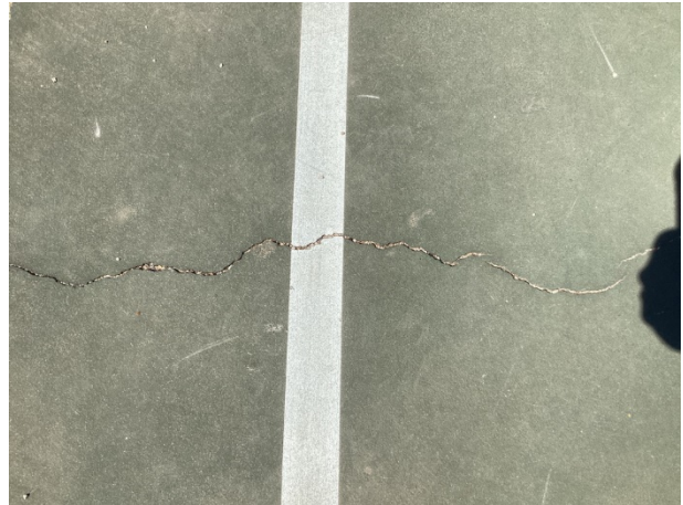
Surface cracks at basketball court
