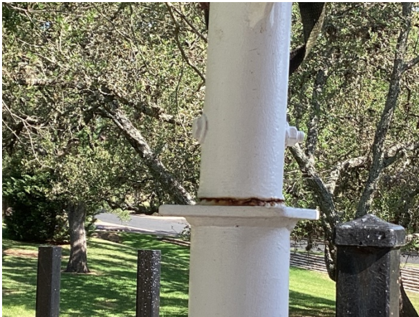
Rust at frame
