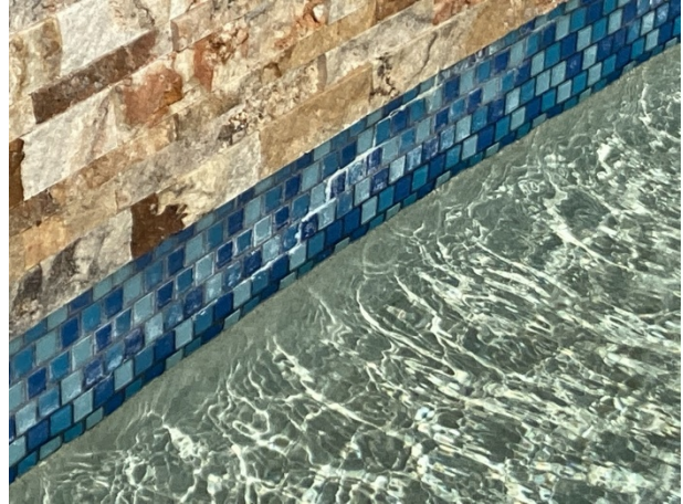
Efflorescence at tile at wading pool
