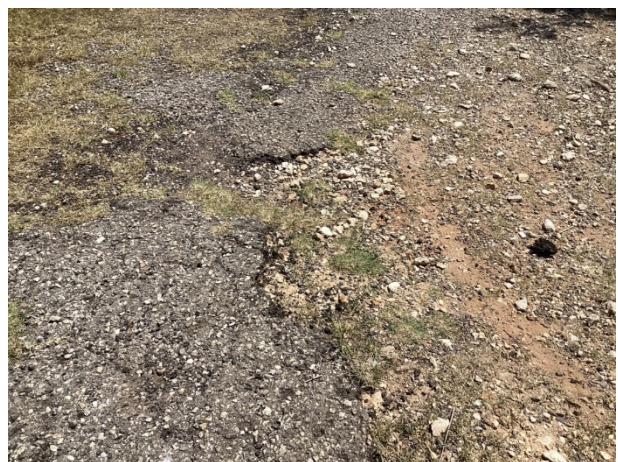
Walking path deterioration
