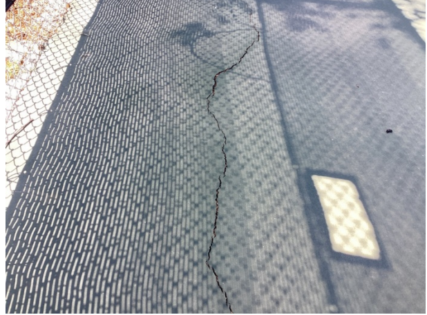
Surface cracks at asphalt tennis court
