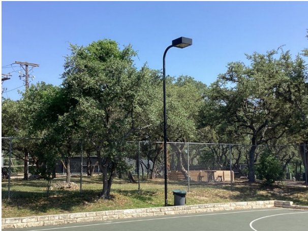
Light pole and fixture
