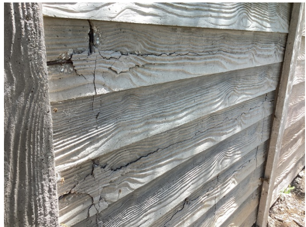
Wall panel cracks
