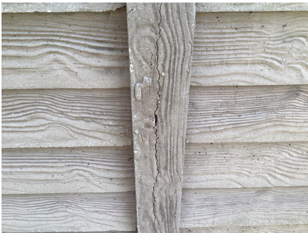
Cracks at column
