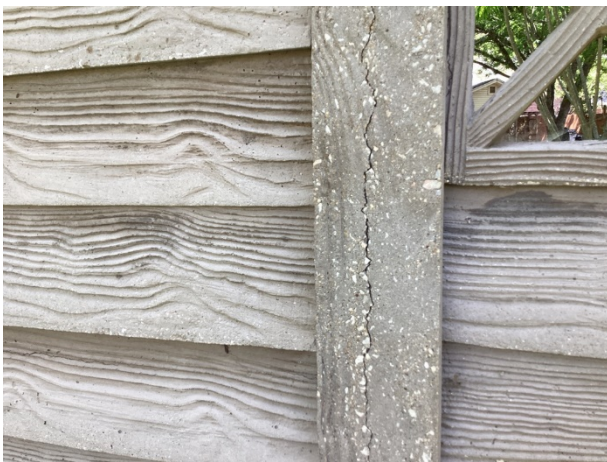
Cracks at column
