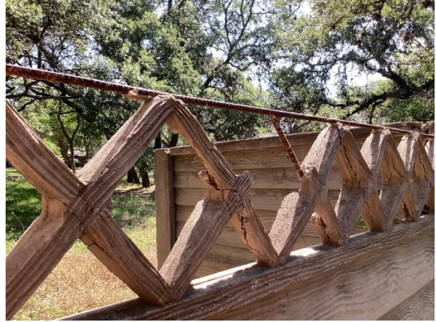
Concrete deterioration and exposed reinforcing steel
