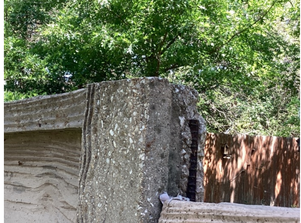
Wall support deterioration and exposed reinforcing steel
