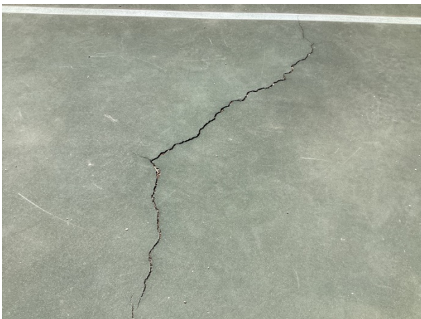
Surface cracks at basketball court
