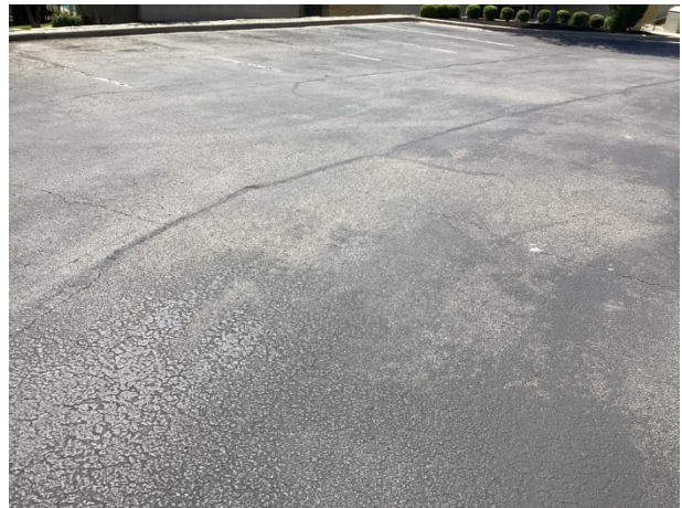
Seal coat deterioration
