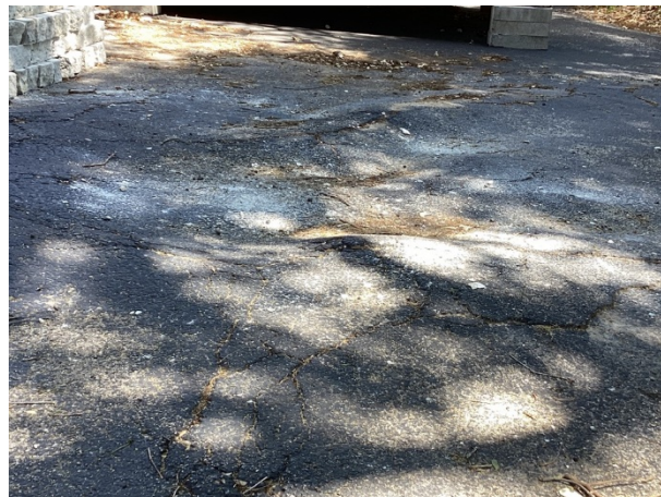
Pavement deterioration by the pool mechanical equipment
