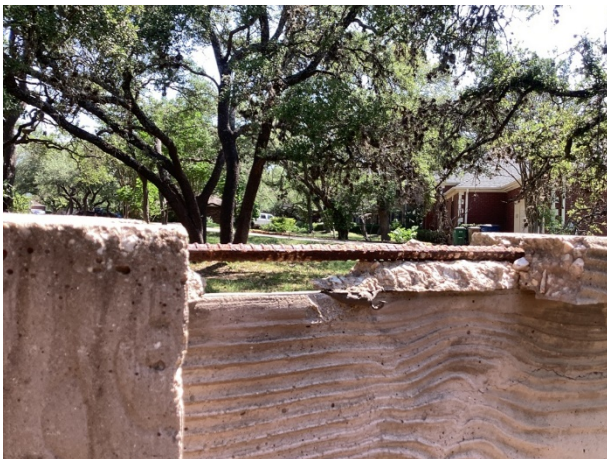
Concrete deterioration and exposed reinforcing steel
