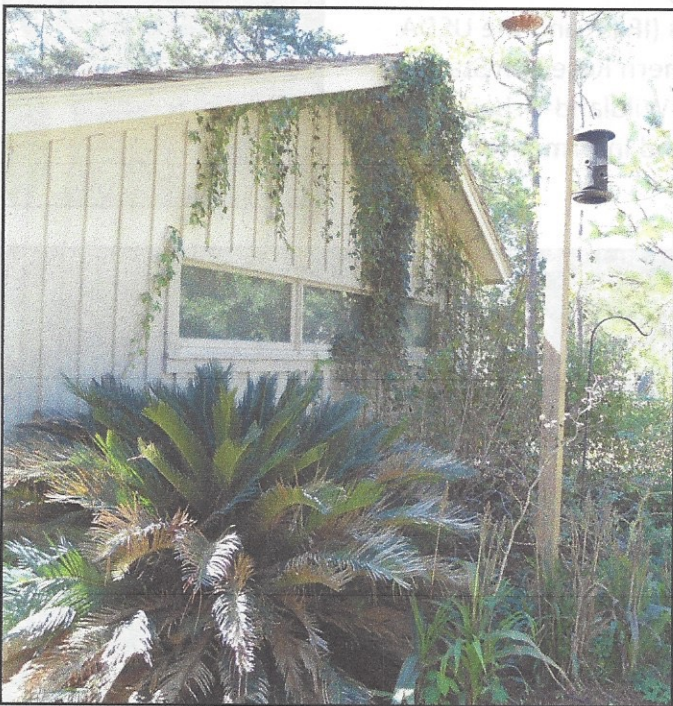
Overgrown vegetation that is within the 30 feet of defensible space can produce significant heat, potentially igniting the home.
